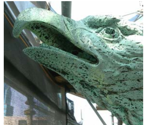
Figure 4. Before Corrosion Removal Process
