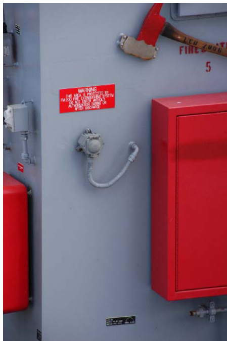
Figure 12 - Electrical Enclosure after 1 1/2 Years (LCU 2006)
