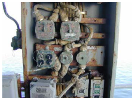
Figure 6 - Corrosion-Prone Stern Gate Controller Area
