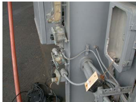
Figure 3 - "Jury-Rig" Solution to Corroded Electrical Box
