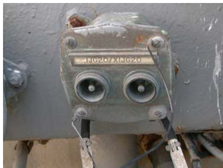
Figure 1 - Corroding Electrical Enclosure
