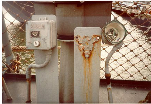
Figure 2 - Ship-Structure Corrosion Resulting from Brass Enclosure
