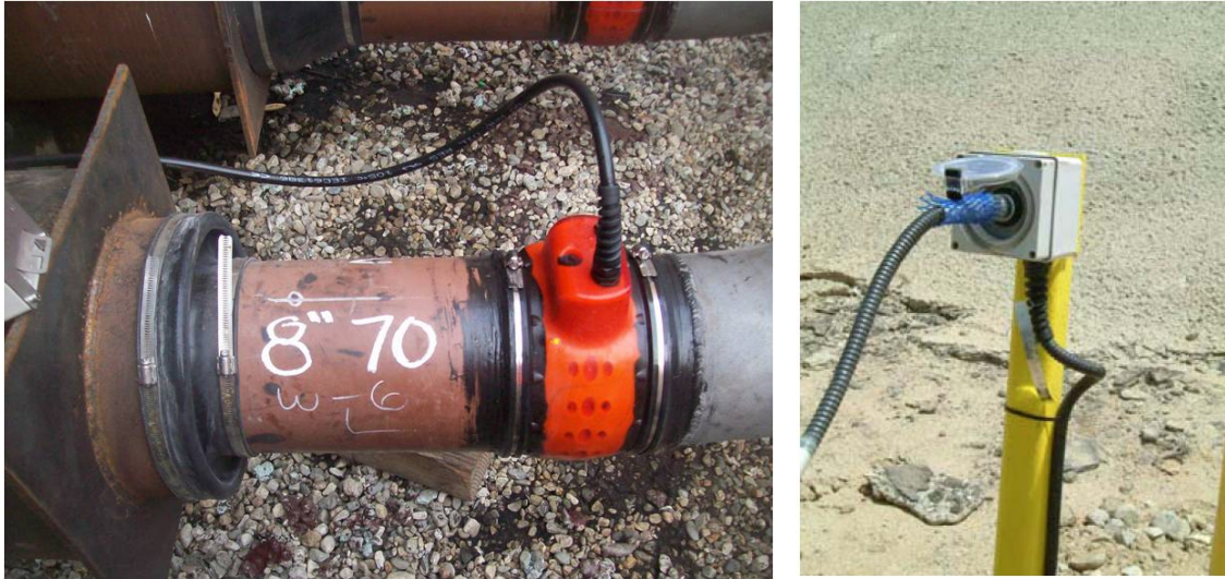
Figure 3: Left, GWUT PIMS collar installed before filling the excavation. Right, PIMS above-ground test point connection.
